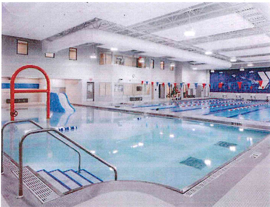
The wall between the lap pool and warm-water pool was demolished to construct a new full-glass partition.
